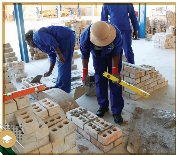
Students applying their brick laying skills during the 2017 "Decade of the Artisan" event
